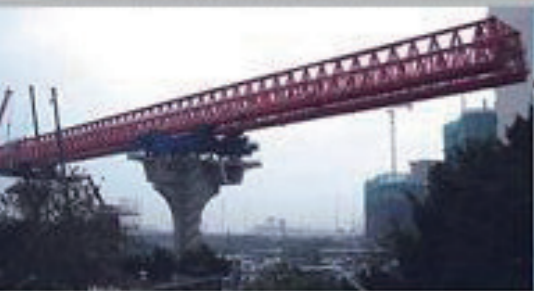
Cantilever Launching Gantry 100 ton, 85m Hongkong Lythee Bay / NESCO
