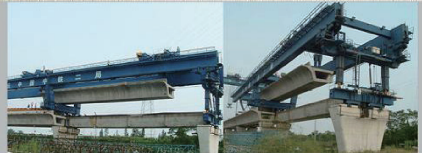
Launching Gantry (450 ton capacity) for GuangZhou-ZhuHai High Speed Railway / 2nd BG CREC
