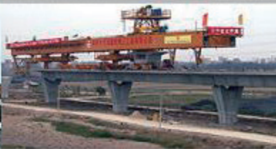
Span by Span Launching Gantry 530 ton, 35m Guangzhou Light Rail No.4 Lot / MBEC
