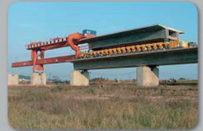
Launching Gantry for going through tunnel (900 ton capacity) for Fujian-Xiamen High Speed Railway / 21st BG CRCC
