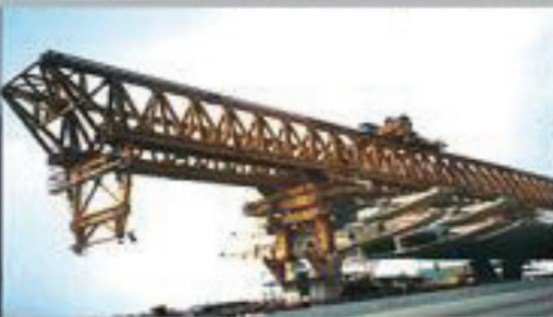
Span by Span Launching Gantry 1600 ton, 38m span Shanghai Humin Viaduct project / FEC
