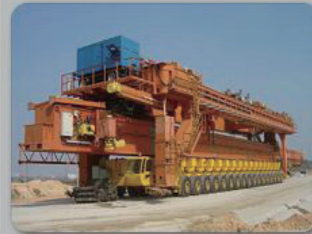
The Launching Gantry is being loaded on tyre trolley for changing jobsite and passing through tunnel
