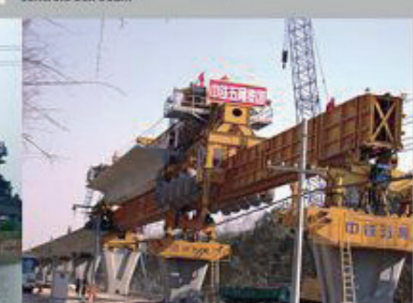
The Special Launching Carrier (400 ton capacity) for the Capital Airport Light Rail Line / 5th BG CREC
