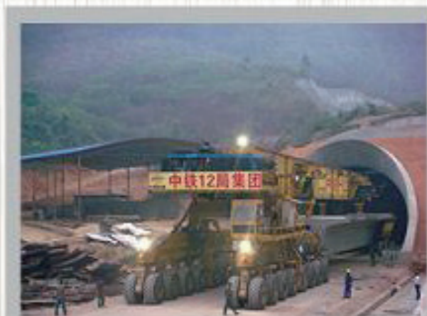
The Special Launching Carrier going through the tunnel with concrete box beam
