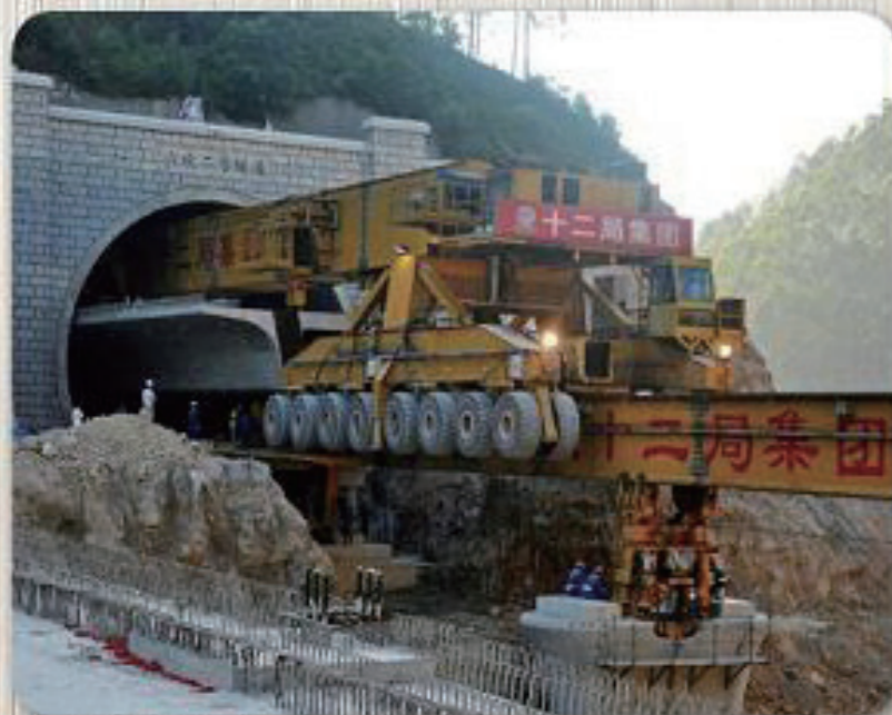
Launching at tunnel portal Special Launching Carrier (900 ton capacity) for LiuZhou-NanNing High Speed Railway 12nd BG CRCC
