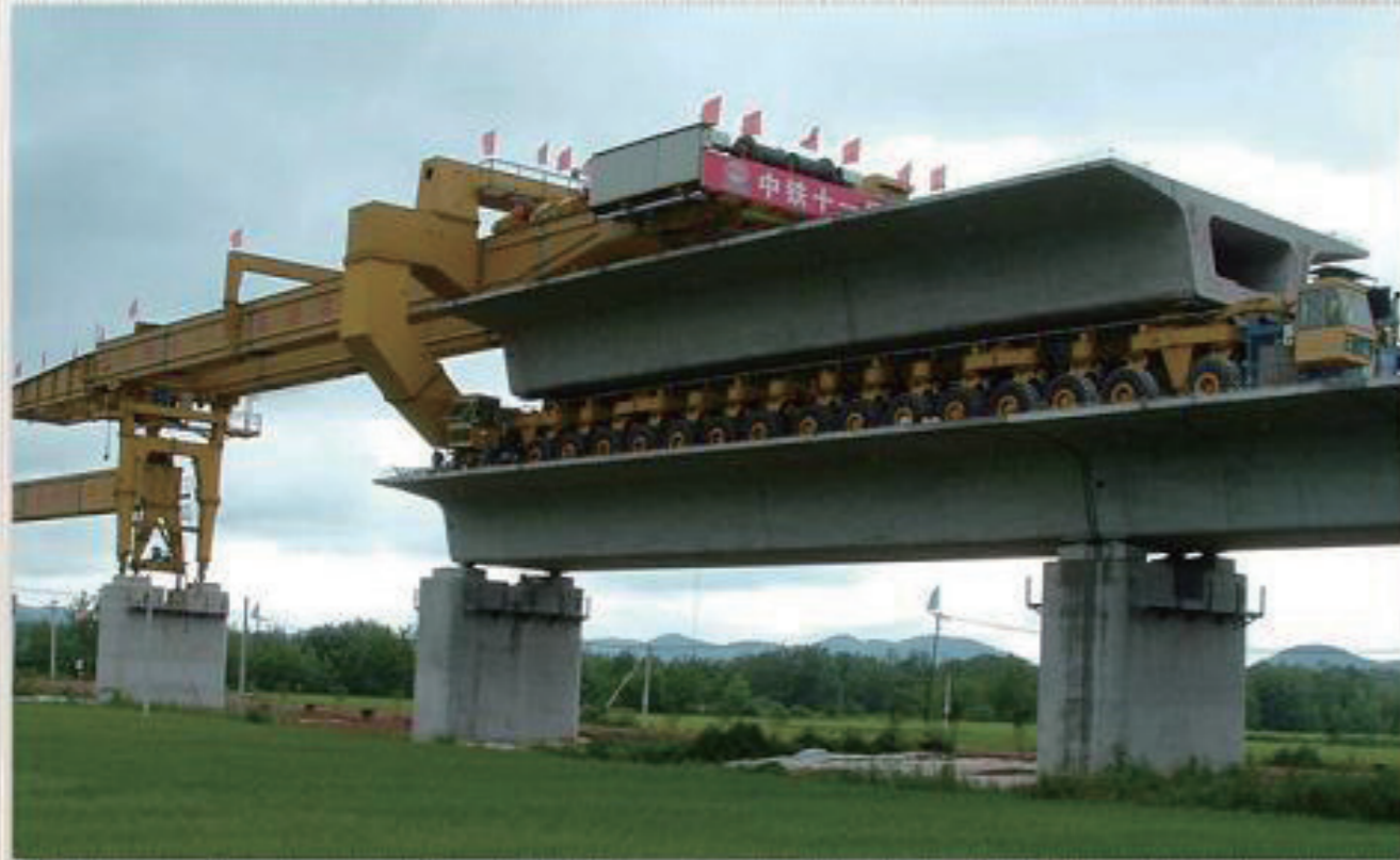
Launching Gantry (900 ton capacity) for WuHan-GuangZhou High Speed Railway / 11th BG CRCC
