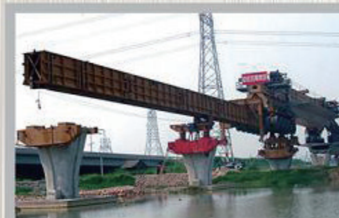
The Special Launching Carrier (450 ton capacity) for Guangzhou No.4 Light Rail Line / 5th BG CREC
