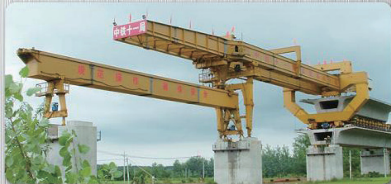
Launching gantry in 900 ton capacity for Wuhan-Guangzhou High Speed Railway/11st BG CRCC
