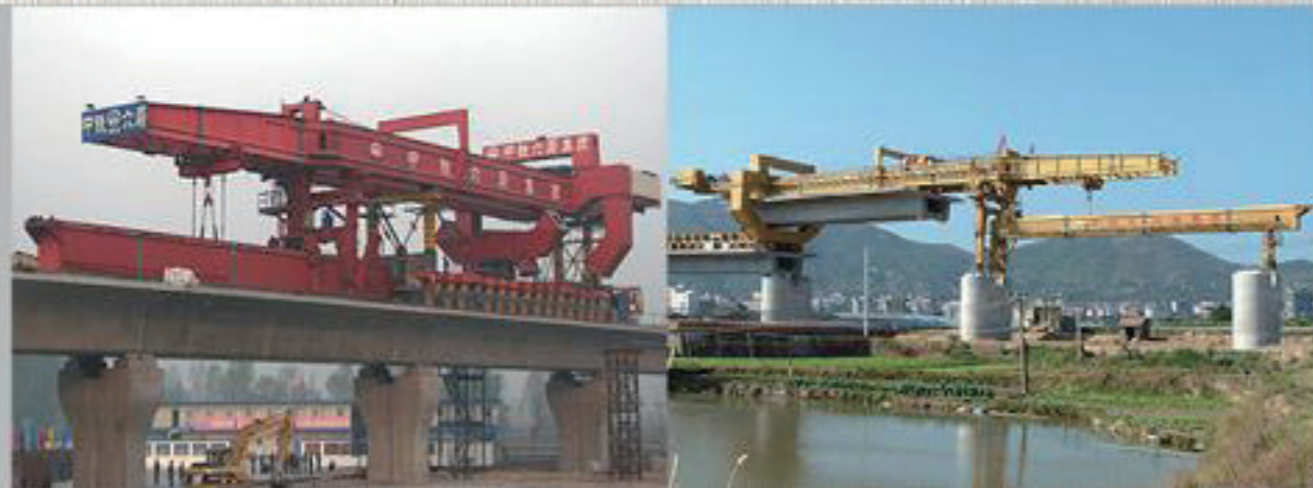
The Launching gantry was loading on tyre trolley for moving from one erecting jobsite to other one Launching Gantry (900 ton capacity) for Beijing-Tianjin High Speed Railway / 6th BG CREC
